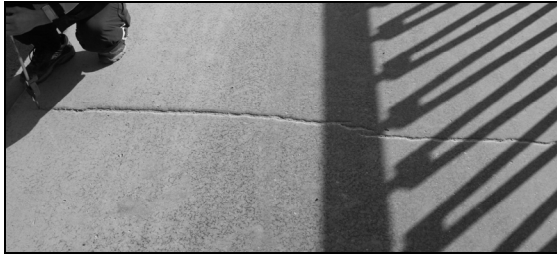
Fig 2. One image of break on the bridge
