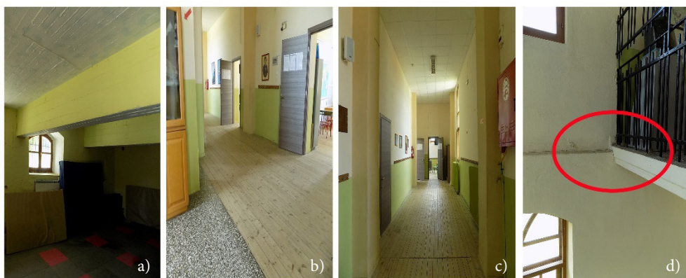
Figure 10. Constructional aspects of the stone school in Arnaia, 1931: a) Concrete slab and beams of the ground floor (image from the basement); b) Concrete slab part and wooden floor of the 1 st floor; c) Consecutive pillars of the 1 st floor; d) Setting of the 1 st floor concrete slab on the wall recession of the ground floor (source: author)
