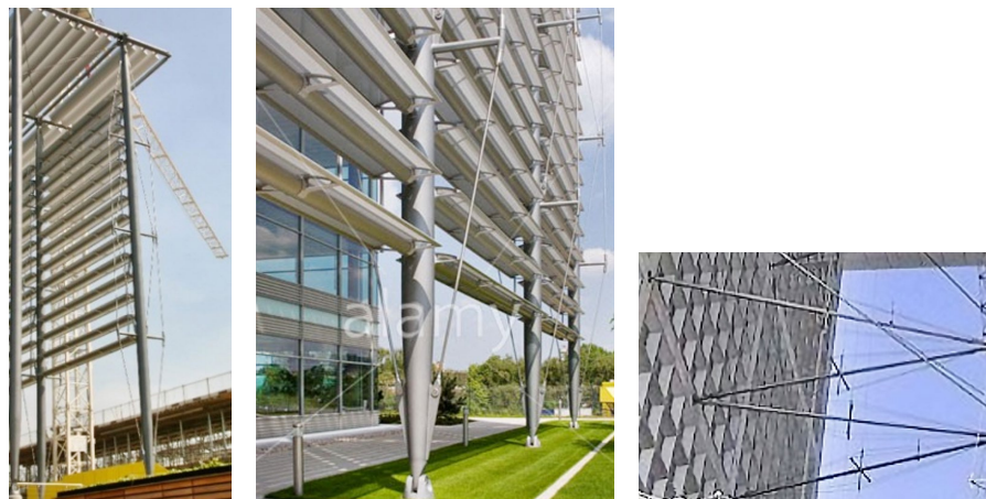
Fig. 1. Stayed members in London (left and middle), supports of Grande Arche lift in Paris
