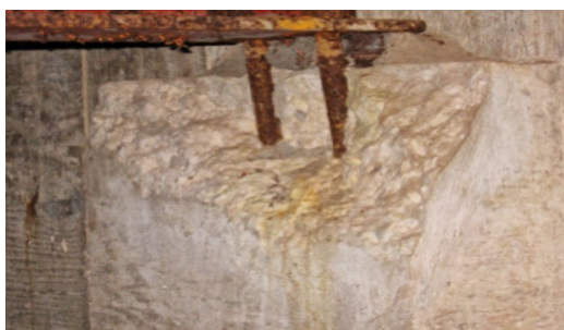
Fig. 4. Expose rebar in CAC foundation
