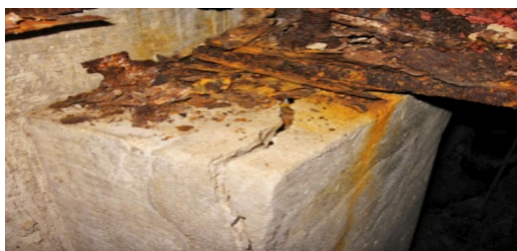
Fig. 5. Damage CAC foundation
