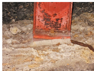
Fig. 8. Bent I-beam supporting column
