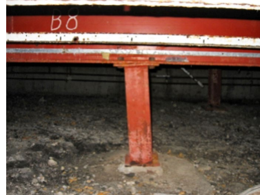
Fig. 7. Bent/shifted CAC foundation
