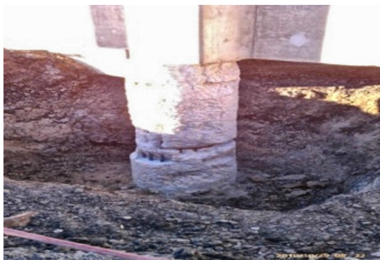
Fig. 11. Exposed rebar in pier
