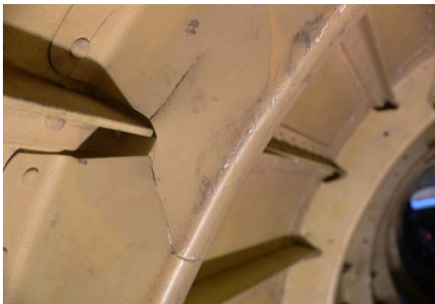
Fig 4. Fatigue cracks in frame as a result of dynamic overload induced by additional concentrated weight in middle part of tail beam
