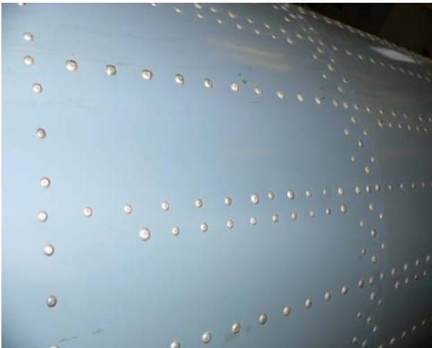
Fig 2. Picture of technological rivet-joint of stringers between frames 7 and 10 (outer view)
